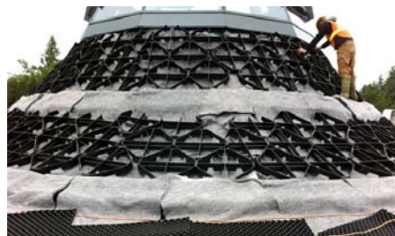
The Floradrain® elements adjacent to the pitched roof area where Georaster® was applied.
