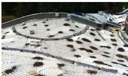
The roof of the visitor centre shortly after the installation of the Floraset® FS 75 elements.
